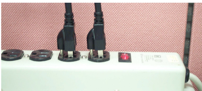
Figure 3.2: Power cord plugs should have same orientation in the socket/ 插座上电源线方向相同 / 插座上的電源線方向應相同
